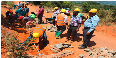
Participants demonstrate construction of galley control during the training on Environmental and watershed management training
