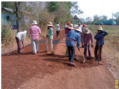
Photos 4: Cambodian workers repair roads as part of the public work program
